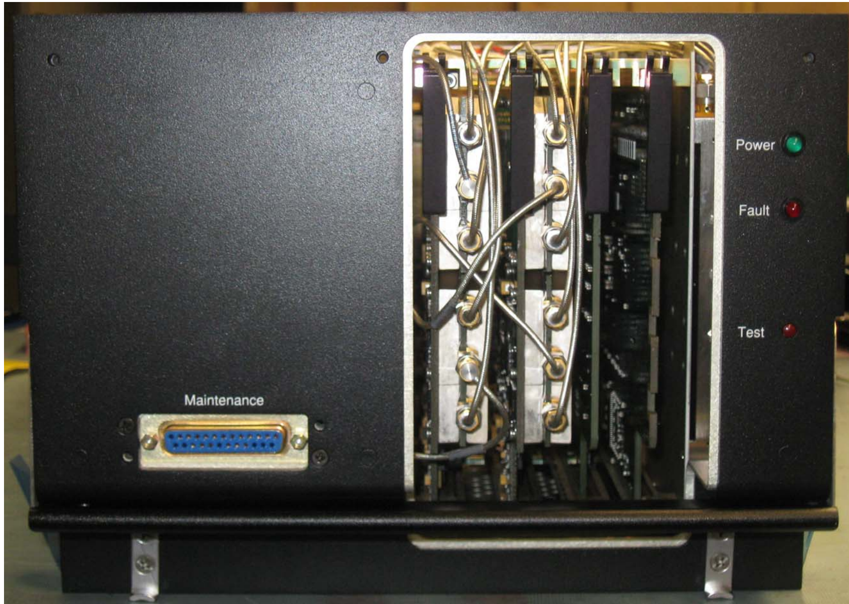
Figure 20: Interconnections Front View
