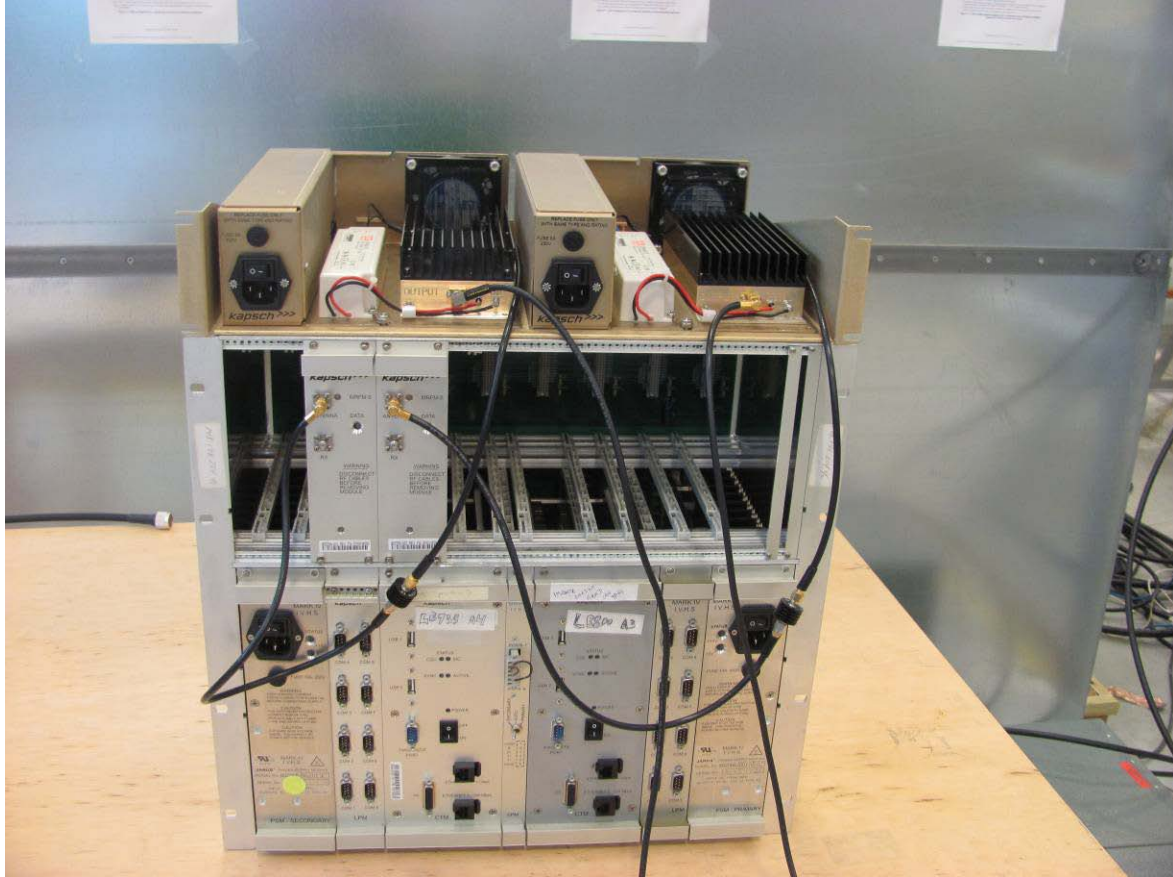
Illustration 6: Two instances of 802295AA were installed in the host.
