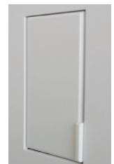
Incorrect: Dimmer/switch is flush with faceplate. Loosen control mounting screws.
