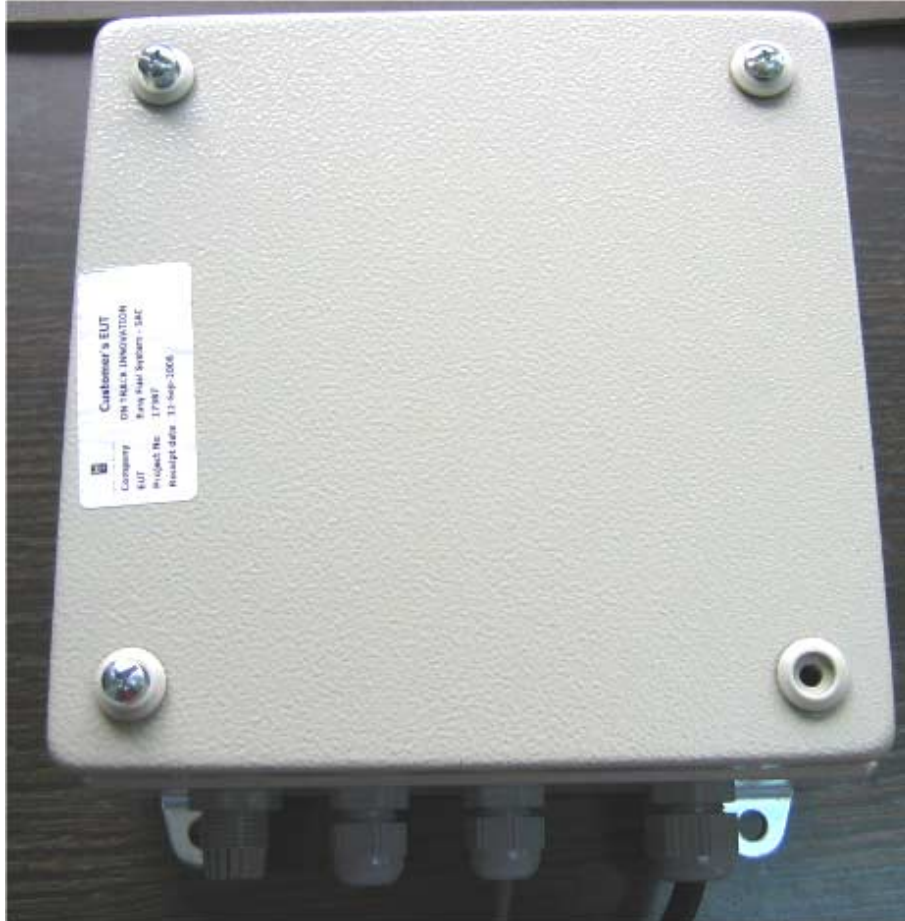
Photograph No.3 Site controller top view
