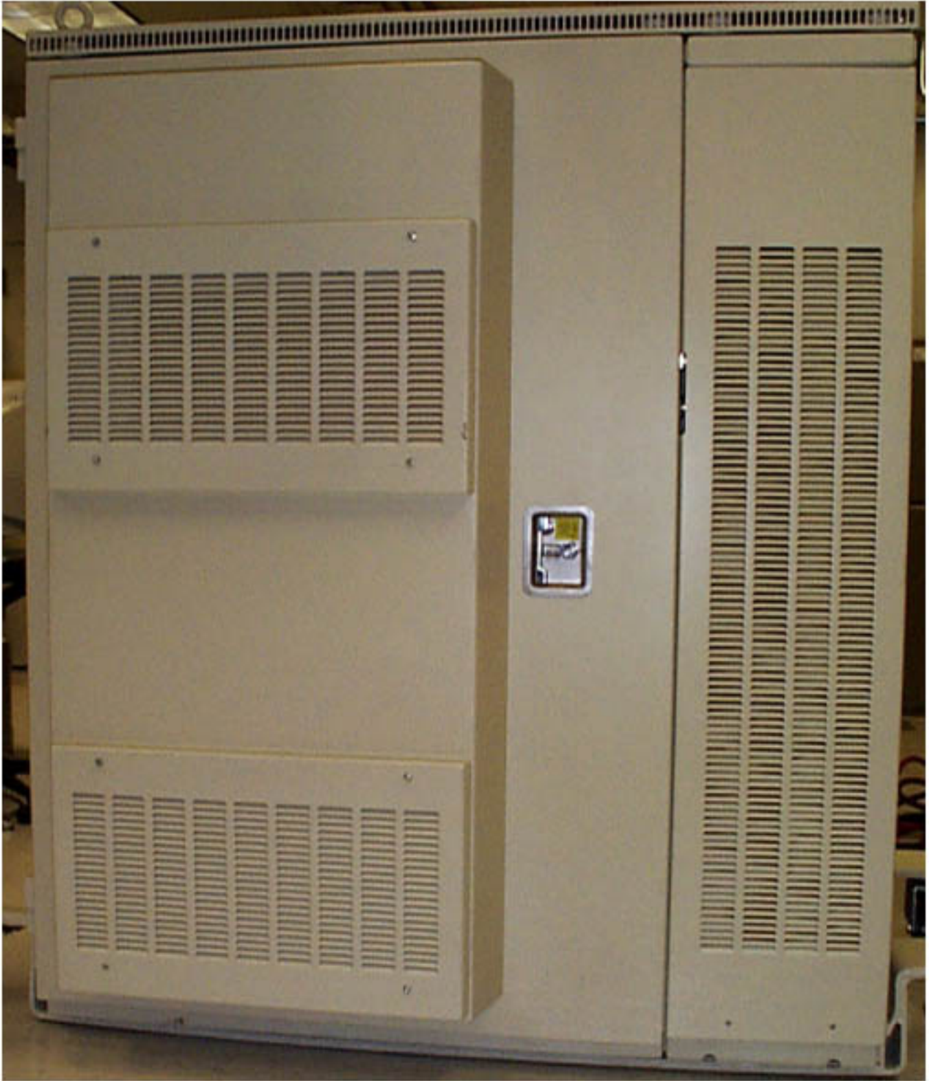
IHET5EG1 SC4812ET 1X/EVDO @ 800 MHz Front View Doors Closed
