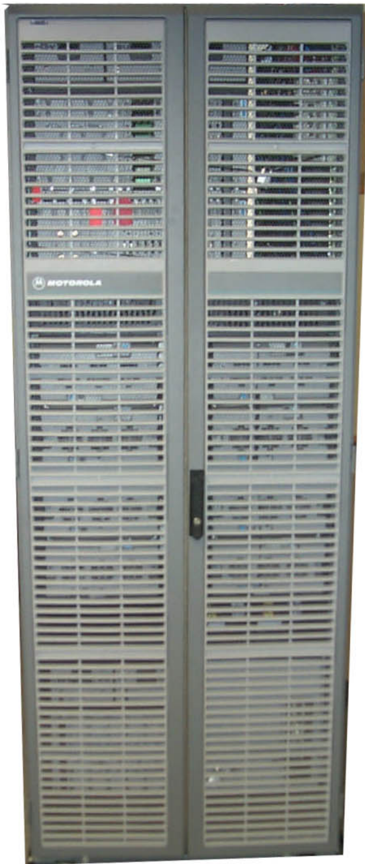
IHT5AW1 -48V SC4812T 800 MHz Front View Door Closed
