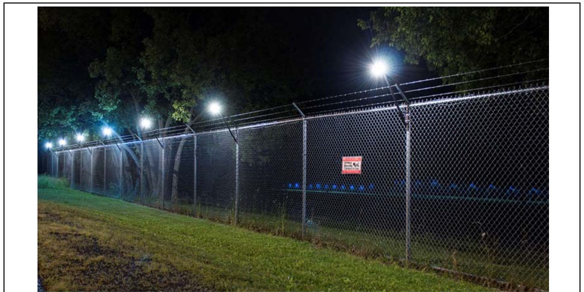
Figure 1: luminaires at night
