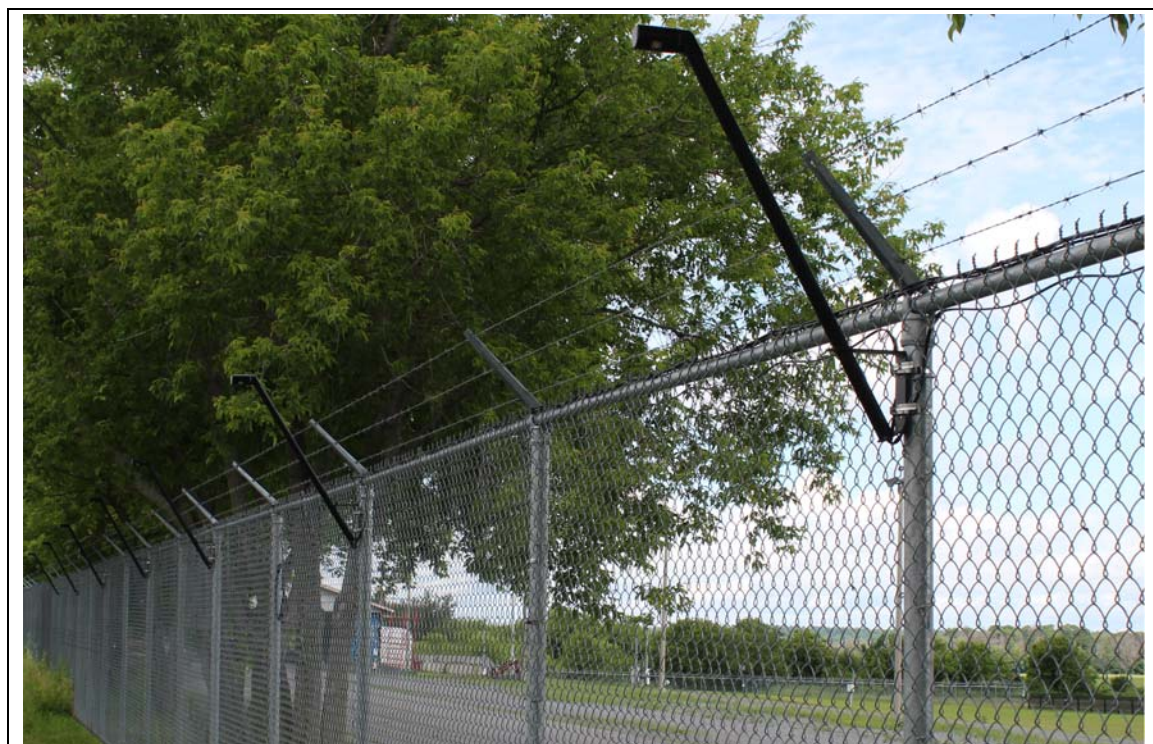
Figure 13: 2.4 m (8 ft.) chain-link fence with luminaires
