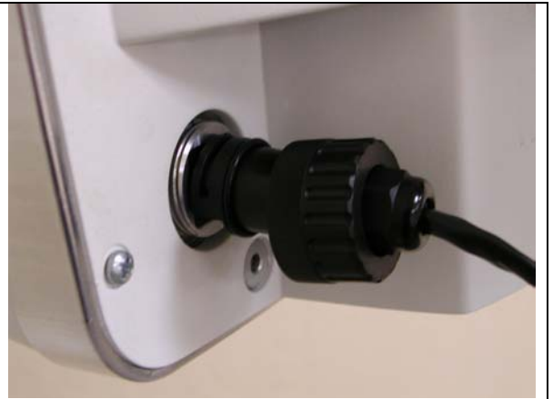
ODU connection not weather secured
