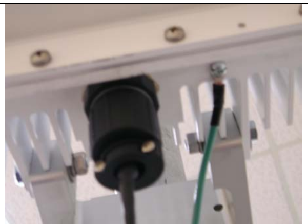
ODU bottom showing ground/earth wiring
