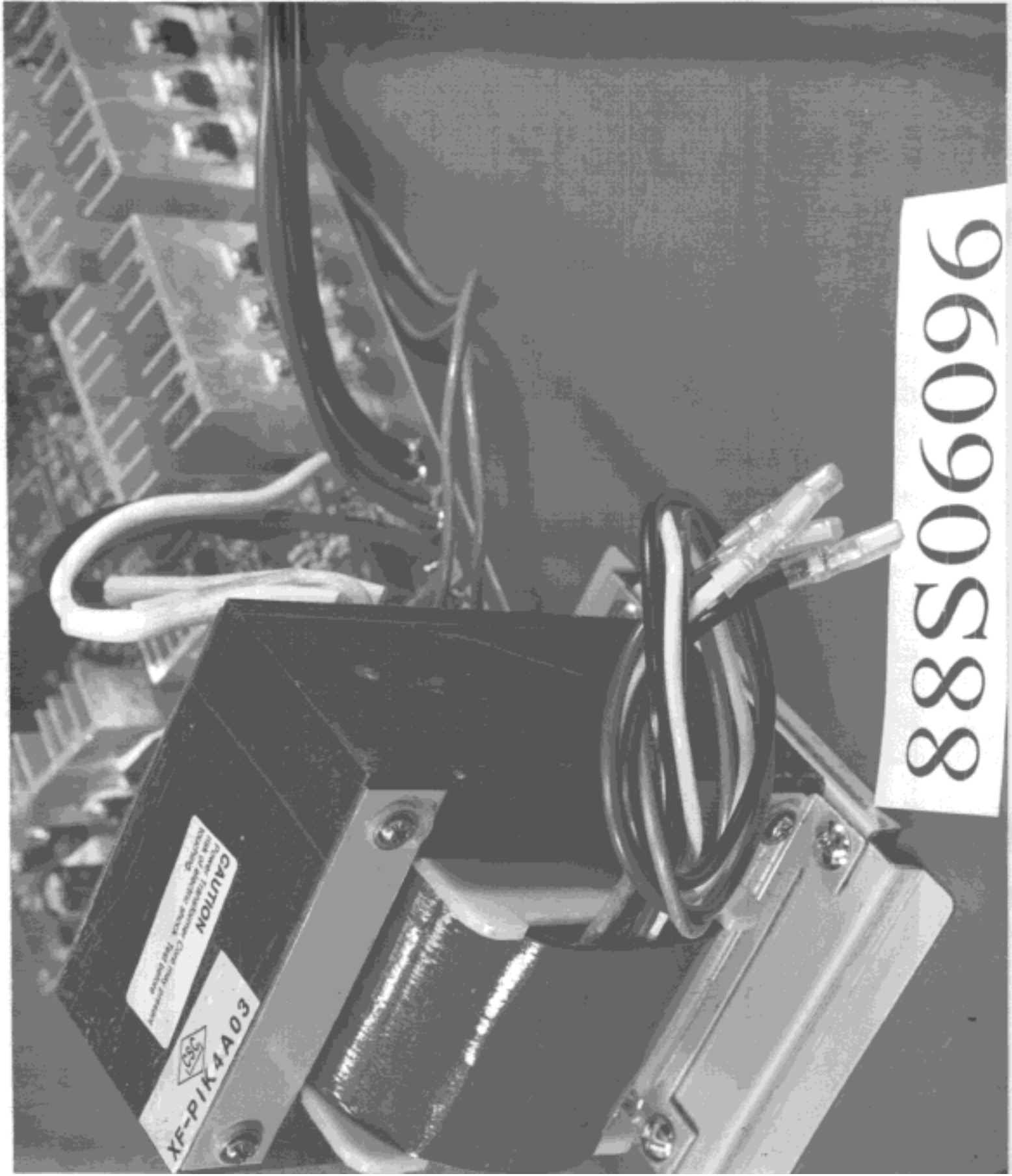
Front View of Power Transformer
