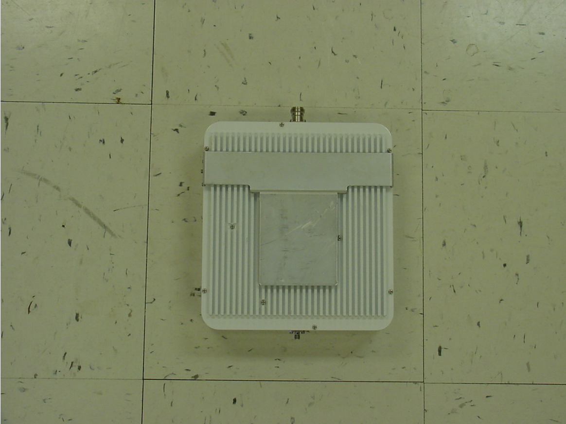
Bi-Directional Amplifier Back View
