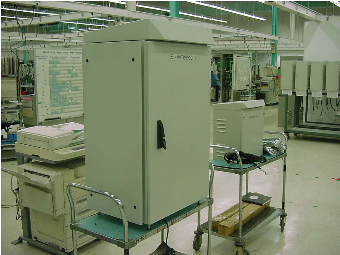
Cabinet Side View 2
