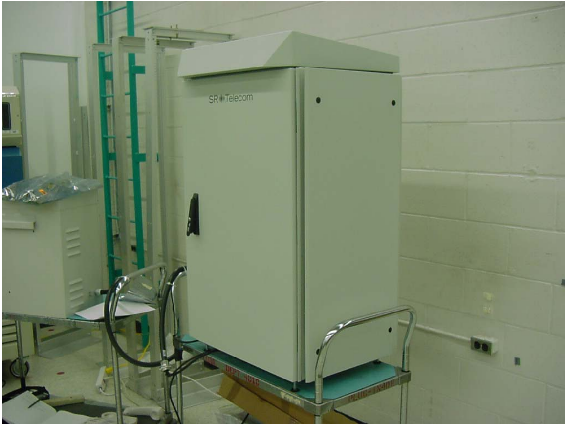
Cabinet Side View 1
