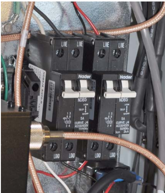
Figure 6: On/Off Circuit breakers.
