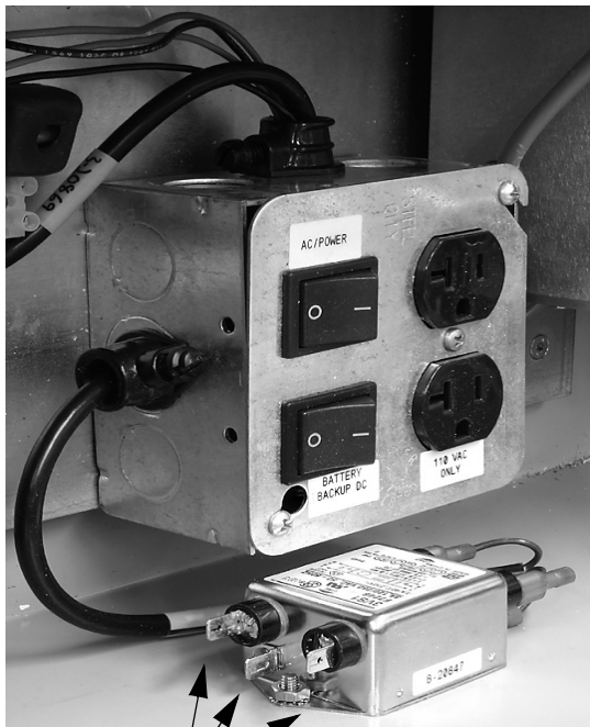
Connect incoming AC line to the input lugs of the AC line filter
