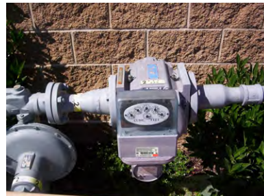
Sensus commercial 500G ERT module mounted on a GE Oil and Gas meter with an instrument drive
