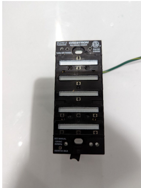
Internal Photograph with coverplate removed
