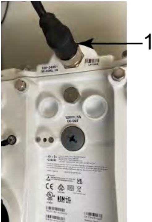
Figure 37 AC power cable connection location
