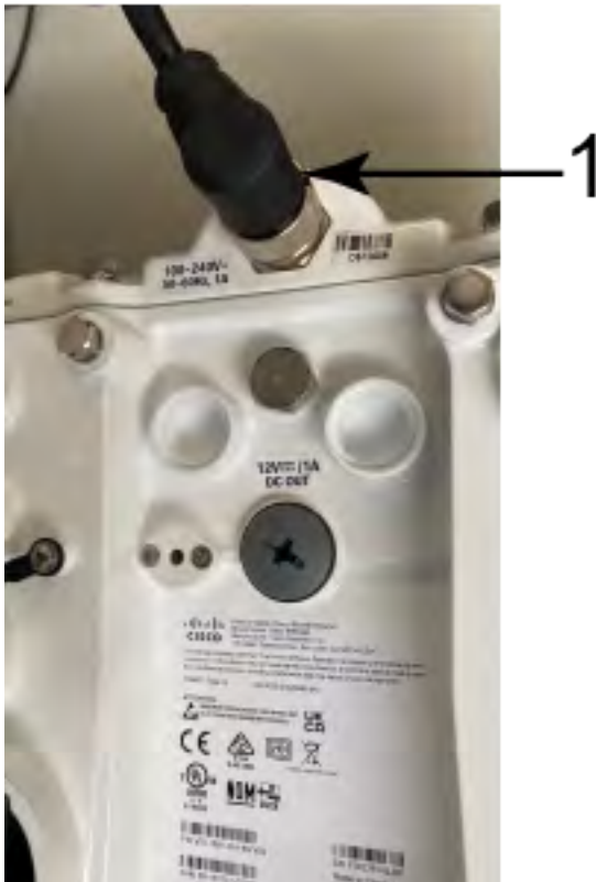
Figure 6 AC power cable connection location
