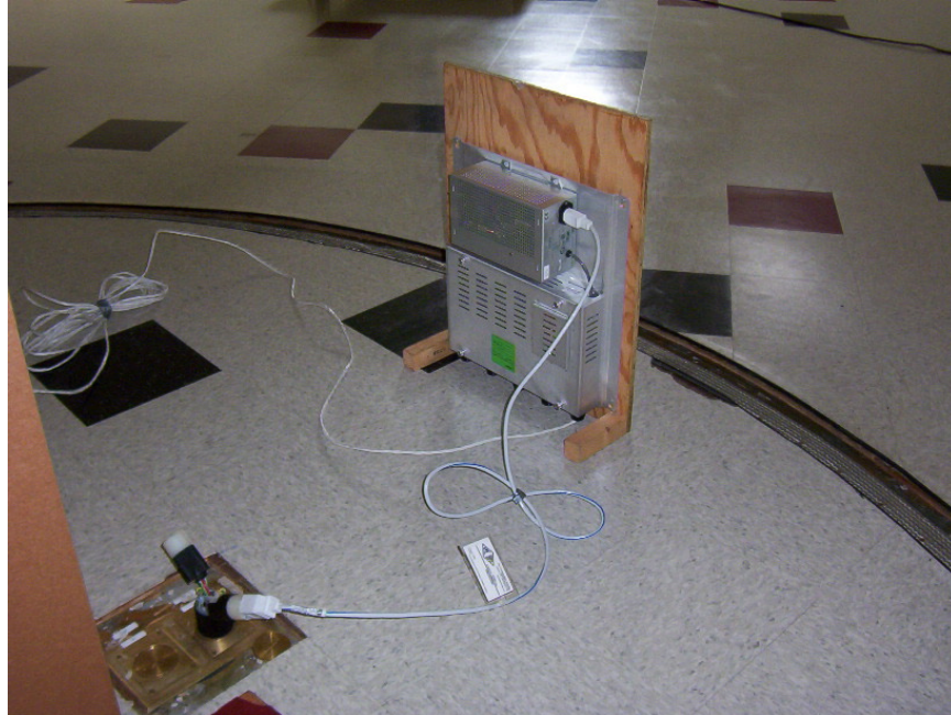
Photo 5 – Detail of Control Module and Cable Layout
