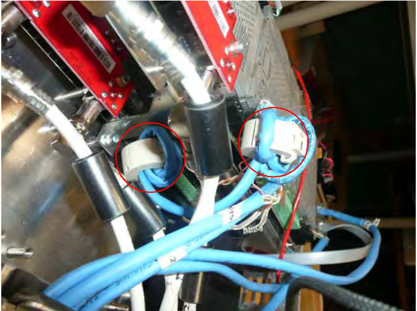
Figure 1 – Fair Rite P/N 0443806406 installed on Sync Cable; Configuration 1
