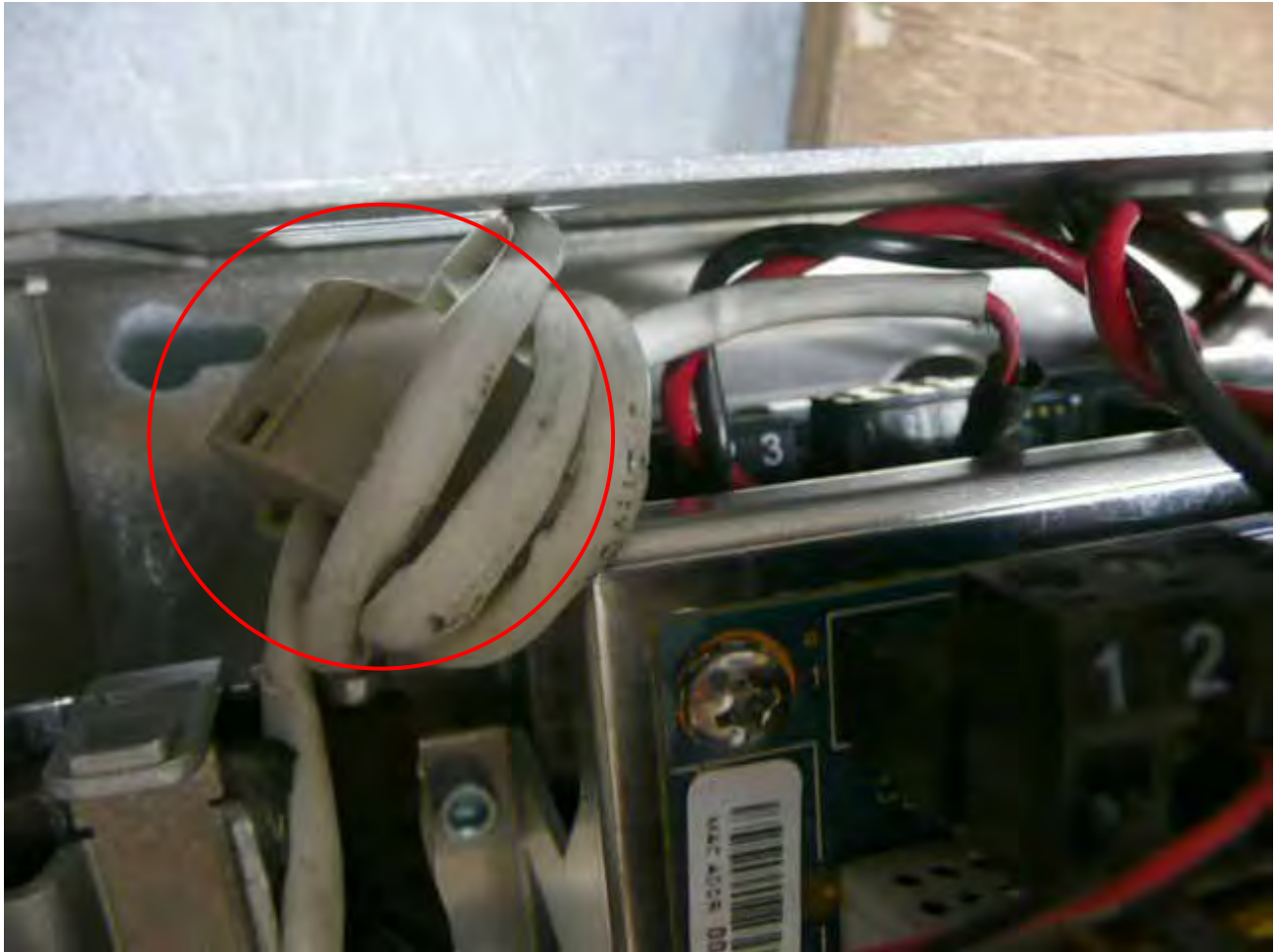
Figure 2 – Ferrite on DC side of Power Supply
