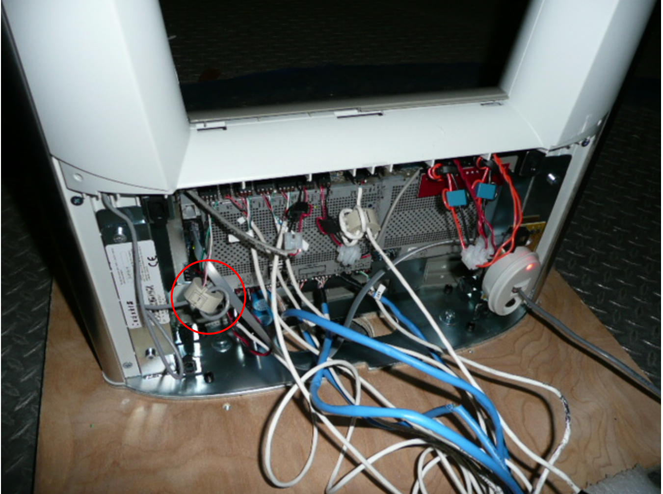
Figure 1 – Fair Rite P/N 0443806406 installed on people counter cable; Configuration 1
