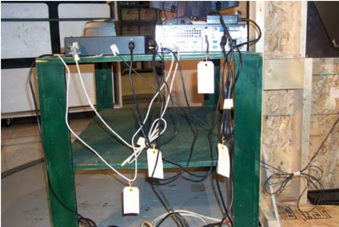
Model 877 Cabling Rear View
