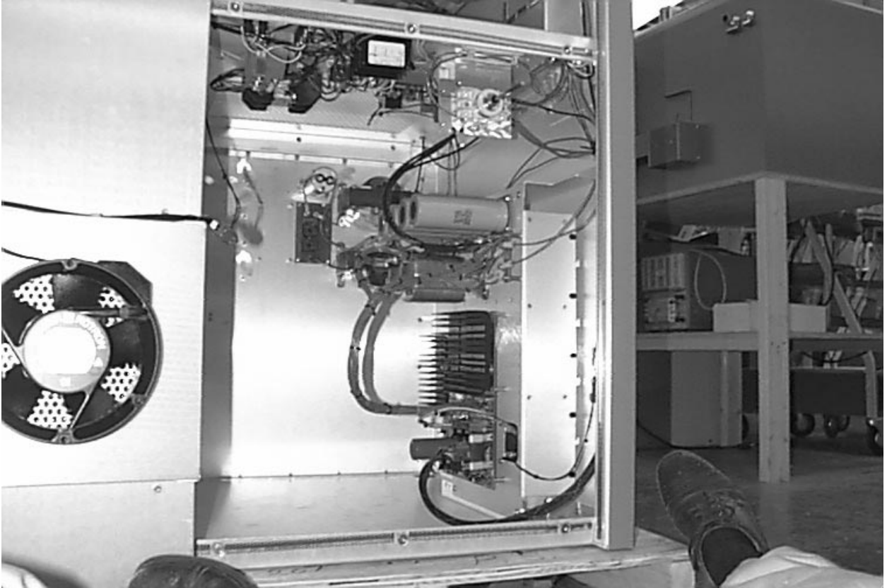
Power Supply/AC Distribution Section
