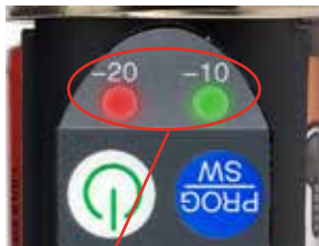
LEDs on control panel
