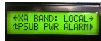
Example of system status with active alarms
