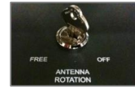
Keyswitch on door of RDU
