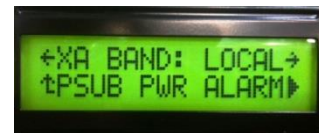
Example of system status with active alarms
