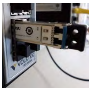
SFP module uninstalled
