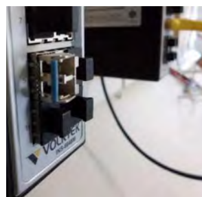
SFP module Installed
