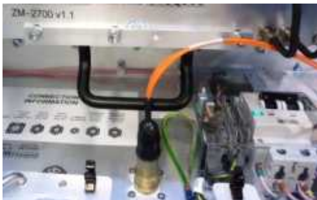
Fibre cable and connector restricting access
