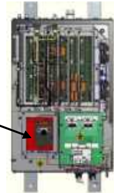
Radar distribution unit
