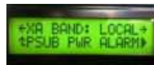
Example of system status with active alarms
