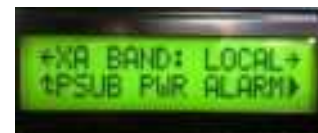
Example of system status with active alarms
