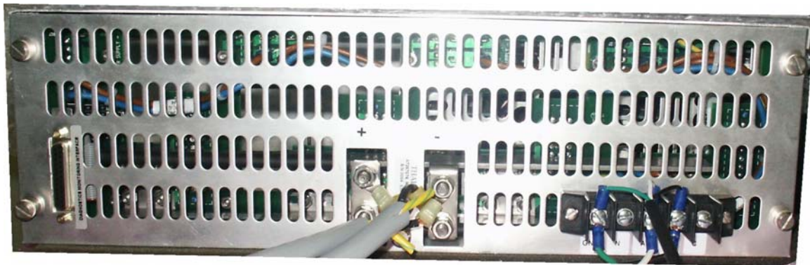
Figure 5 Front-end 48VDC rectifier system (rear view)
