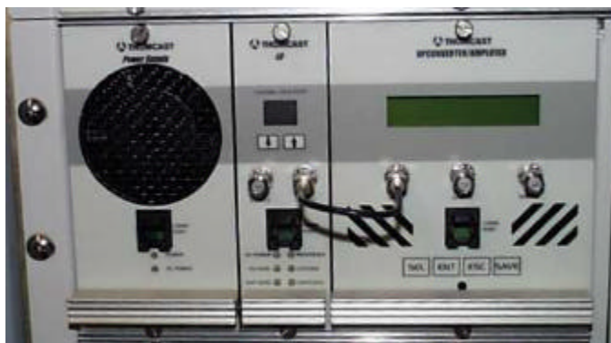
Figure 1: Cabling the LO signal.
