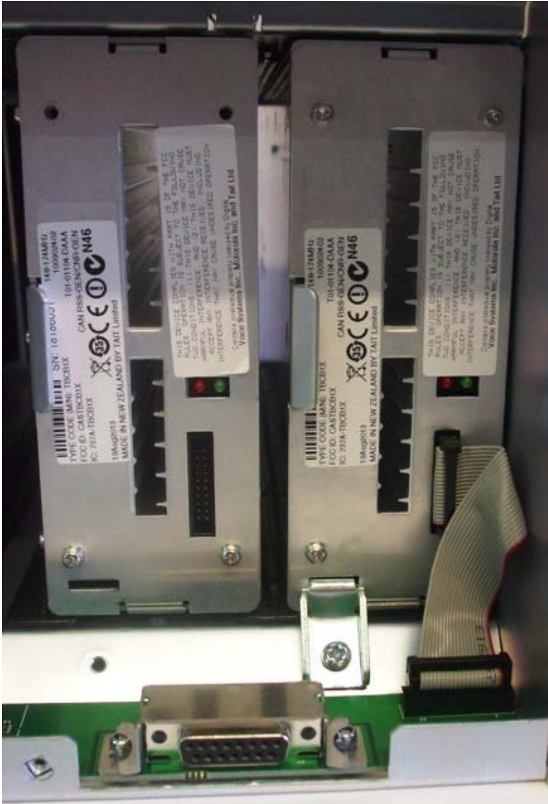
2 x receiver modules in the rack front view
