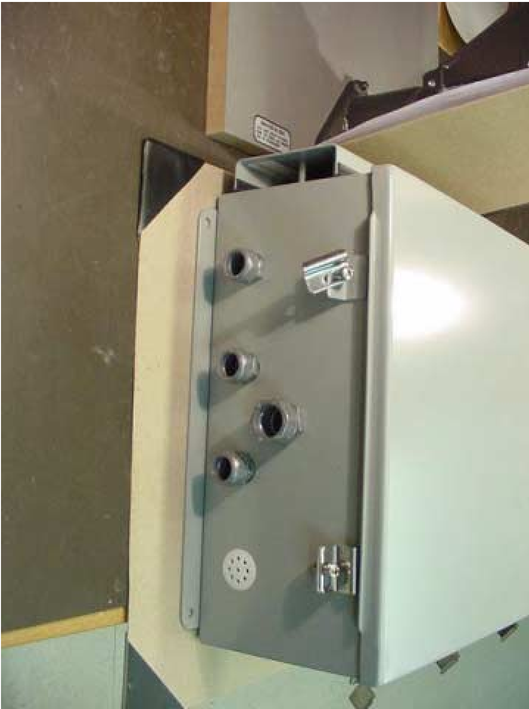
SIDE OF CASE WITH CONDUIT FITTINGS
