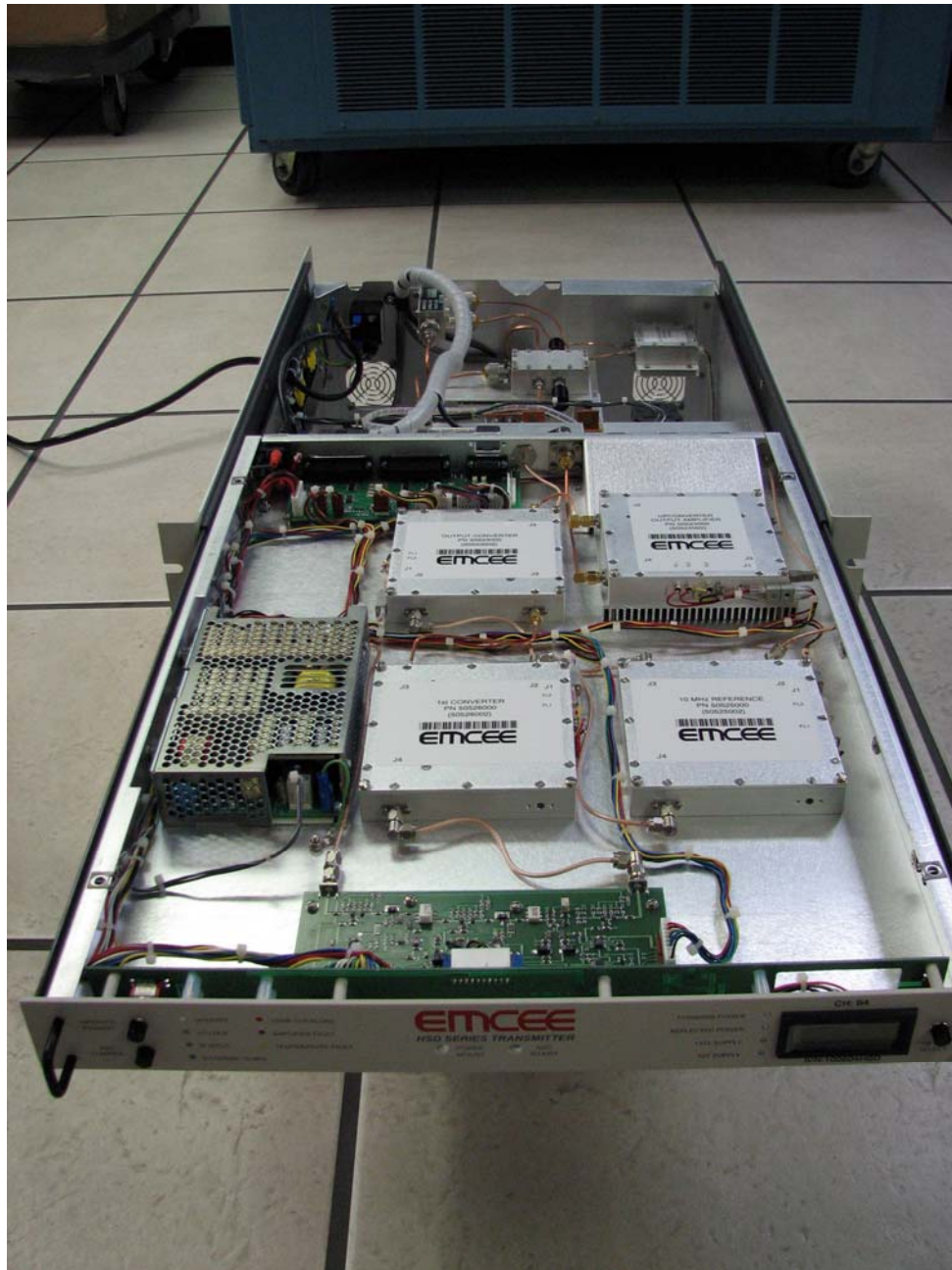
HSD Chassis Service Access
