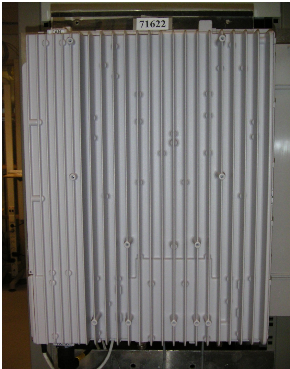
PHT/71622JD21/002 RBS2308 Cabinet with Shields Removed. Front View
