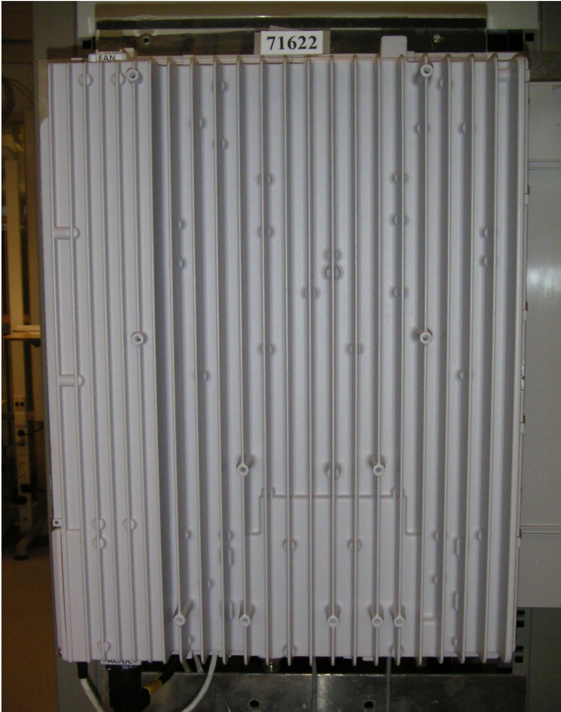
PHT/71622JD11/002 RBS2308 Cabinet with Shields Removed. Front View
