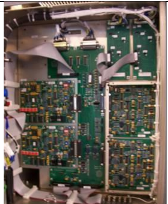
Fig 2.4 Exciter Chassis with PDM Driver Cover Removed.
