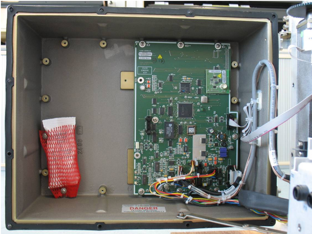
Photo No. 7: Controller board
