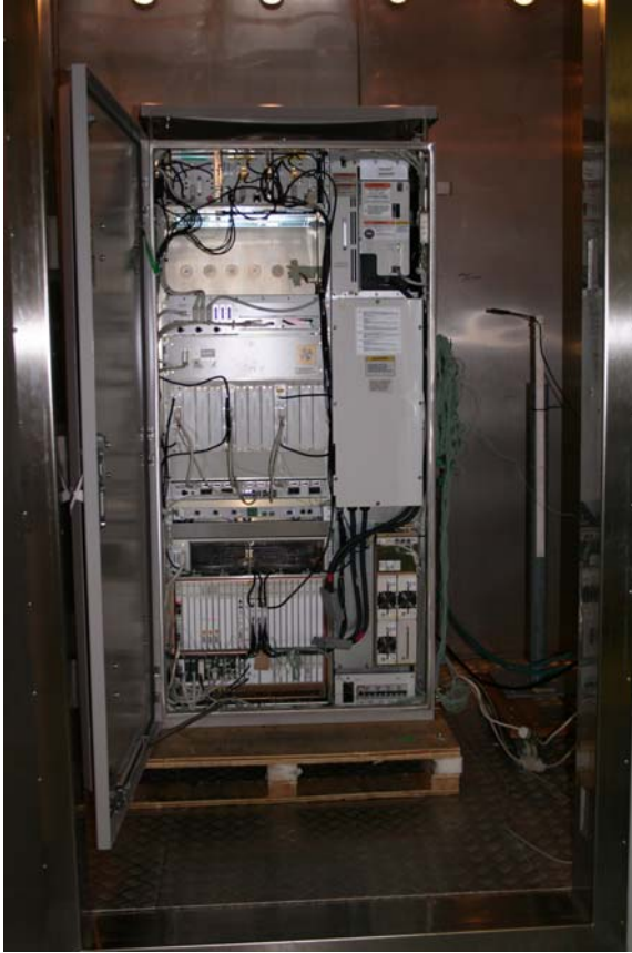
Figure 4 Open BTS under Test
