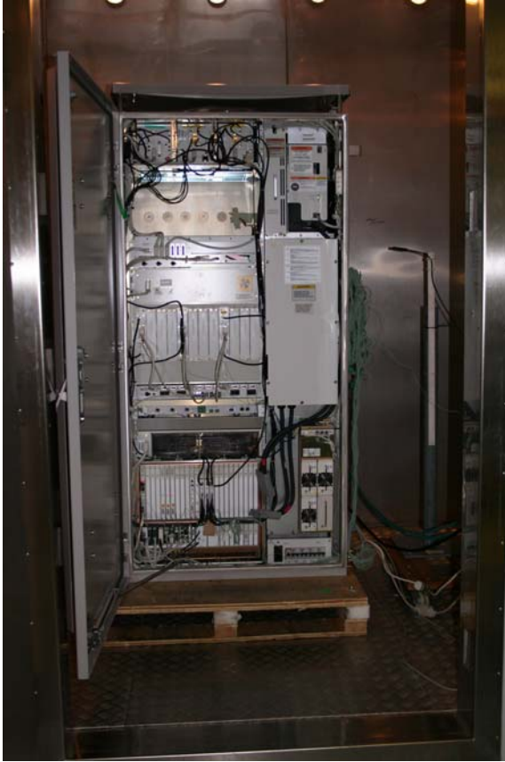
Figure 4 Open BTS under Test
