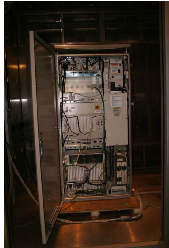
Figure 4 Open BTS under Test
