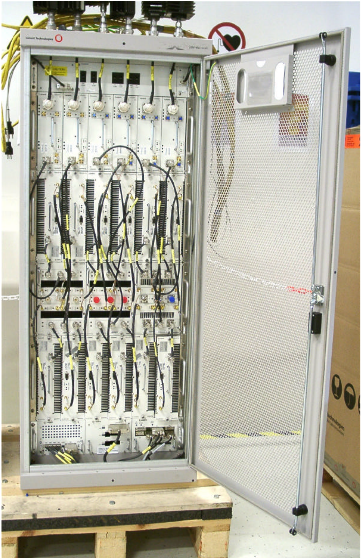
Photograph of twelve TRXHP19 installed in a Flexent Macrocell Indoor cabinet
