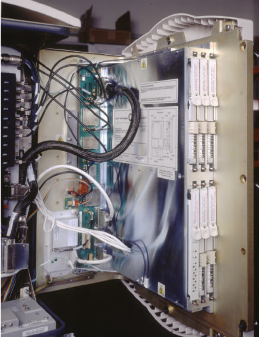
FLEXENT™ Cellular TDMA/Analog Microcell J41698B-1: Interior View Showing Radio Shelf and TOM
