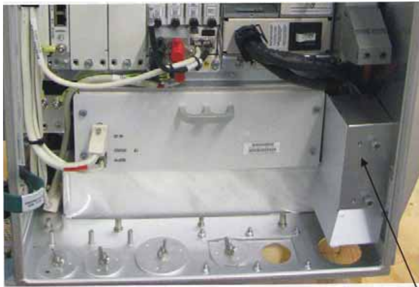
AC Terminal Block Cover (bottom right of BB cabinet)
