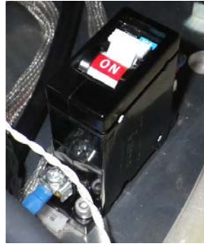
Antenna rotary motor switch "ON"
