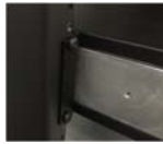
Figure 1b: Rack installation
