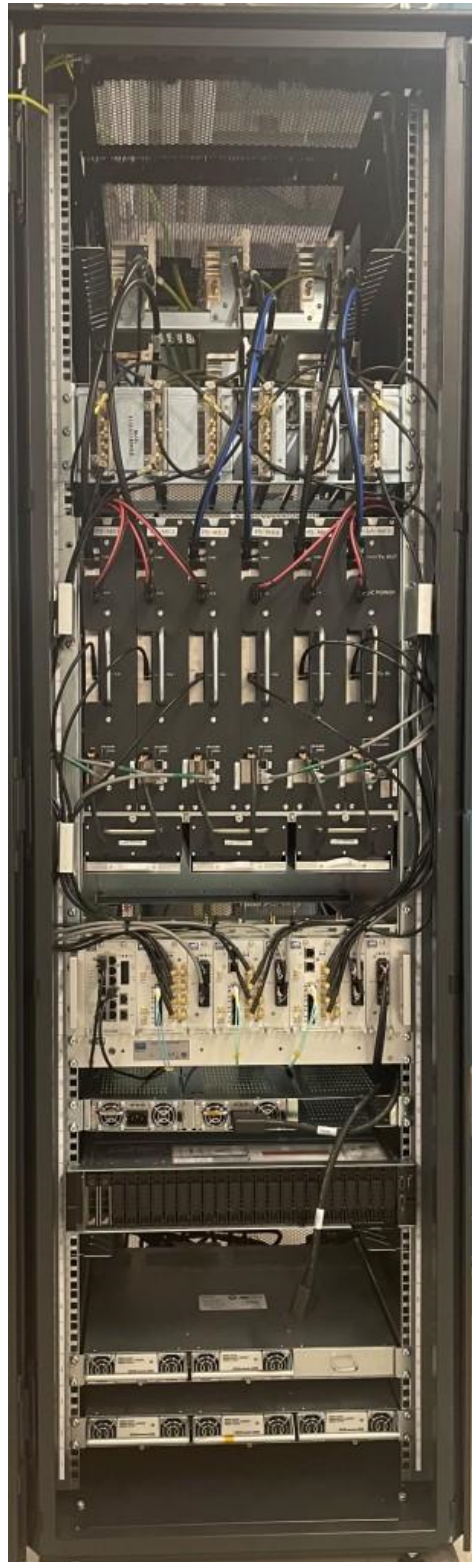
D1-1 External Front View of Cabinet
