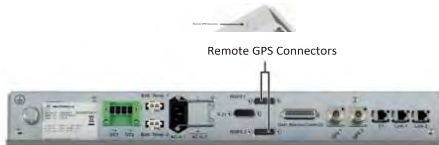
Figure 67: Remote GPS Receiver Connection on MTS 4 Junction Panel
