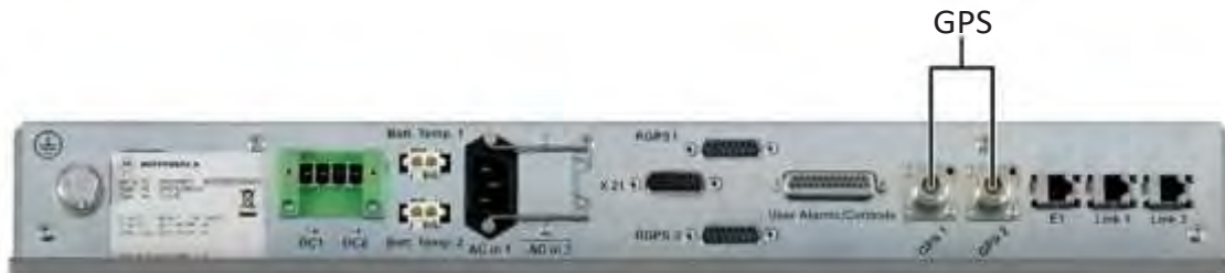
Figure 73: GPS Antenna Connection on MTS 4 Junction Panel
