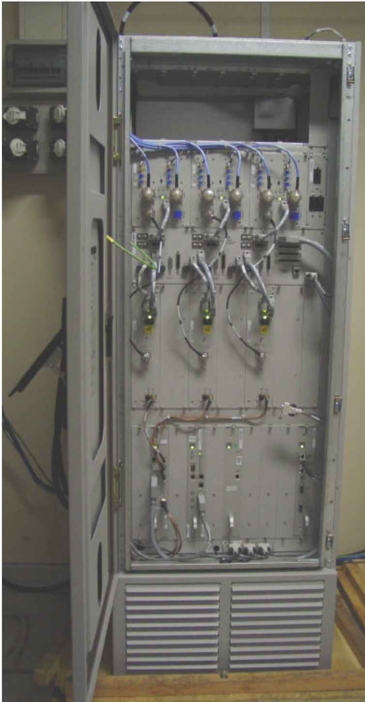
Figure 2: UMTS 1900 Front view with door open
