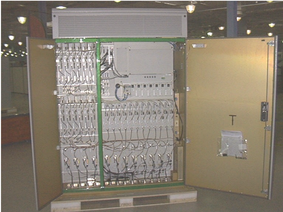
Figure 6 – S12000 Outdoor Front View with Doors Open
