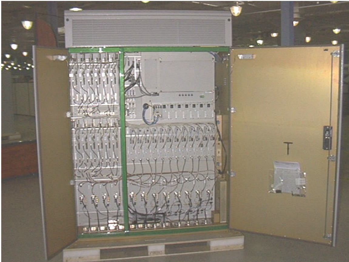
Figure 6 – S12000 Outdoor Front View with Doors Open
