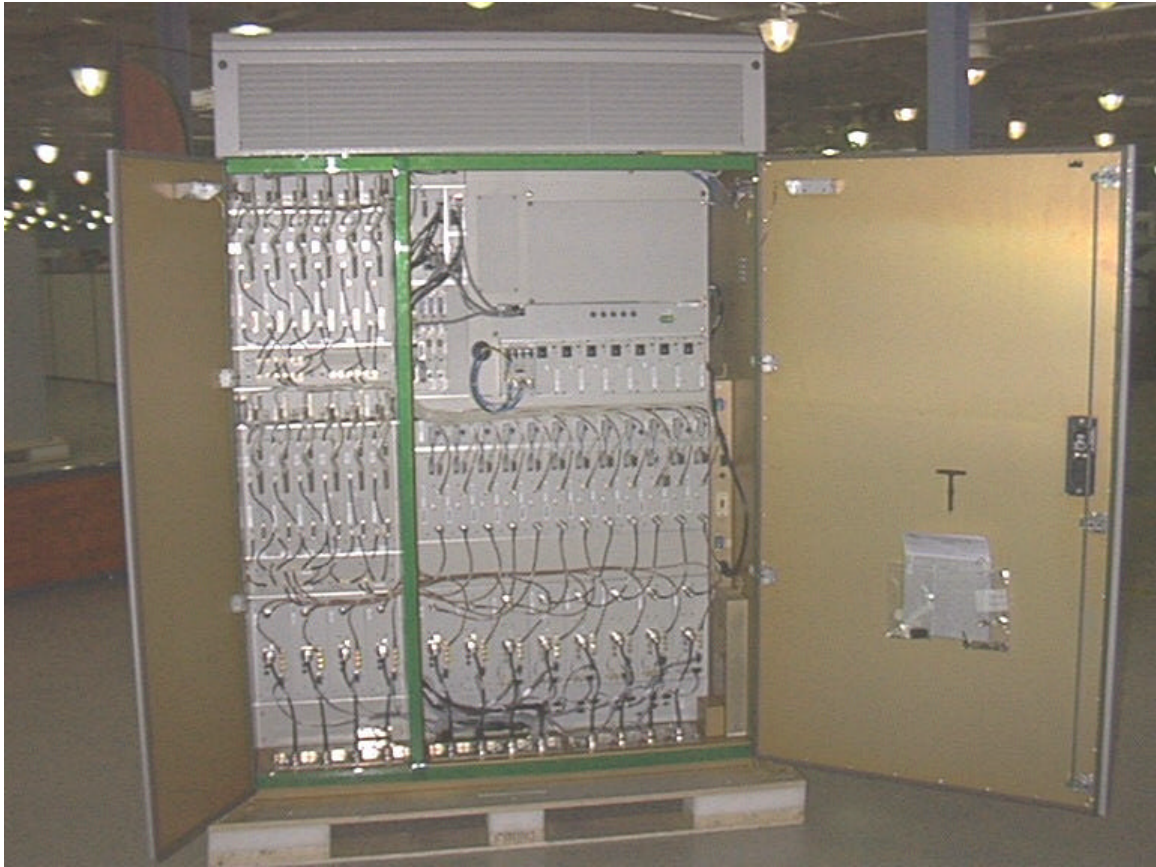
Figure 2 – S12000 Outdoor Front View with Doors Open
