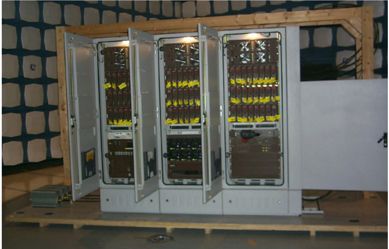
Figure 2: Doors Open Front View of TDMA 800MHz Enclosure System
