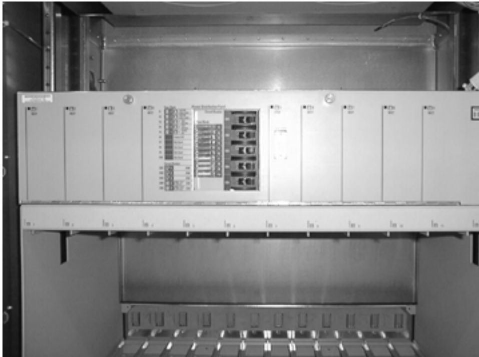
Figure 26 Rectifier shelf - cover closed
