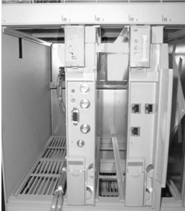
Figure 35 Global positioning system timing module (GPSTM)
